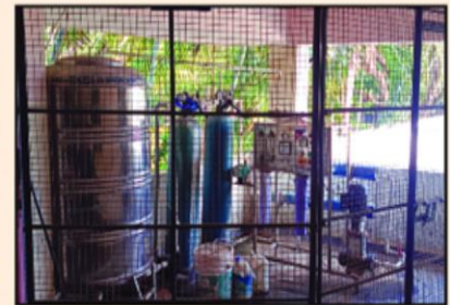
RO Water Plant Facility
